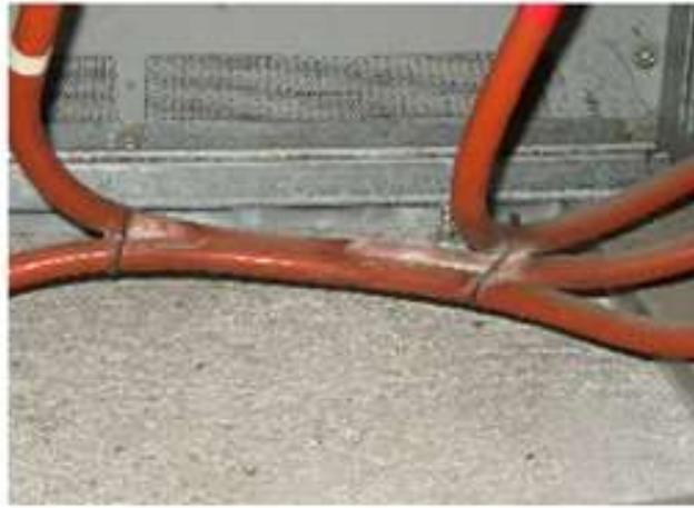
Figure 6: Dust deposit on tie- wrapped cables [16]
