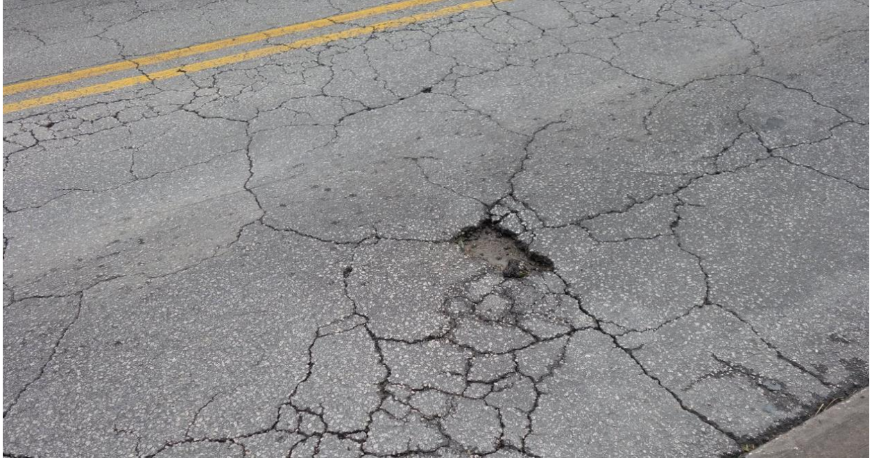
Figure 2 Early-Stage Pothole Development with Surrounding Alligator Cracking on the Sabha–Ash-Shuwayrif Highway, Libya, Representing a Critical Target for AI-Based Predictive Pavement Management.
