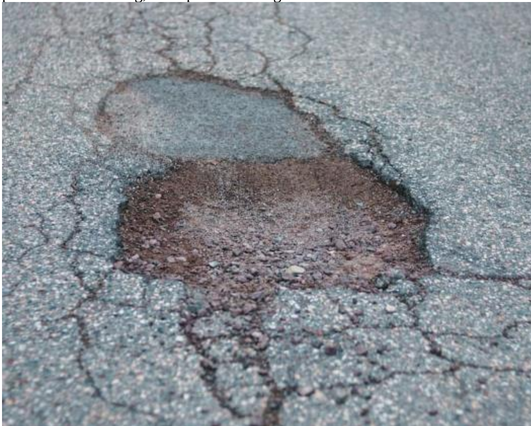
Figure 1 Typical Pothole Formation Following Progressive Asphalt Pavement Degradation
